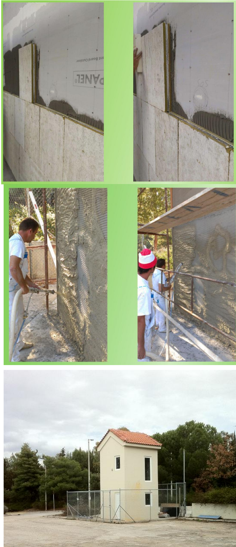
Figure 2-4: Completed installation of new sandwich panels with VIP at the mock up at the NTUA Campus.
