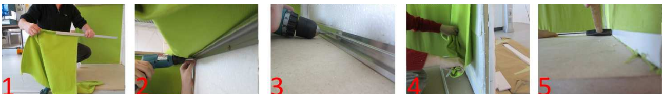
Fig. 11: Sequence of assembling: 1- Inserting fabric with Keder in the upper profile, 2- Fixing the upper profile, 3- Fixing the lower profile, 4- Fabric tensioning, 5- Fabric fixing.
