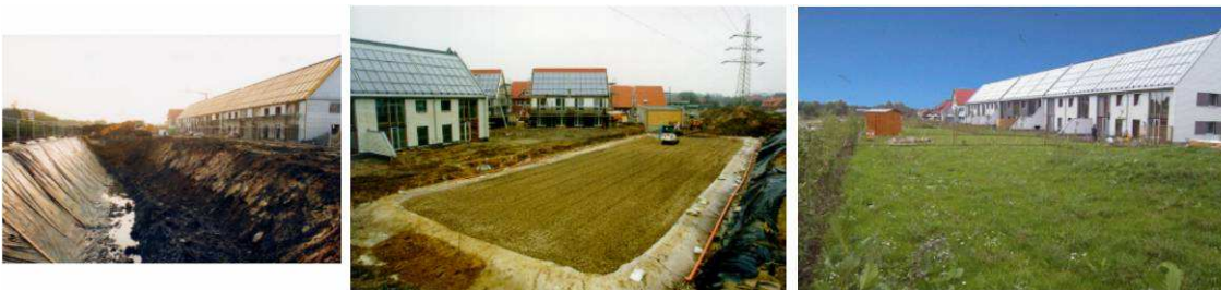
Figure 62: Example of a GWTES realization in Steinfurt, DE, with from left to right: excavation of the storage volume, filling of the storage pit with gravel and heat exchanger mesh and fully covered thermal energy storage [24].
