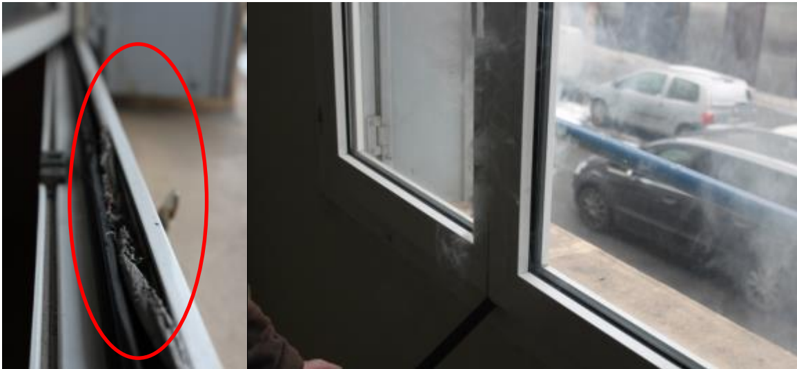
Figure 66: Damaged seals leading to leakages highlighted with the smoke generator (before refurbishment)
