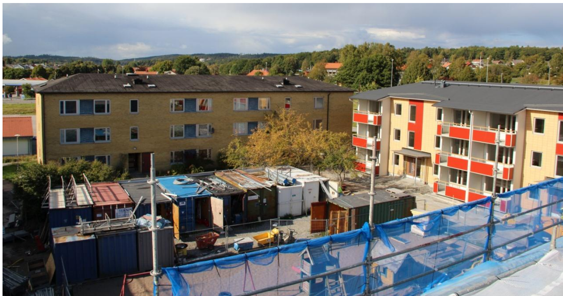
Figure 8 Retrofitting of the last court – buildings before, after and during intervention (source: Skanska)
