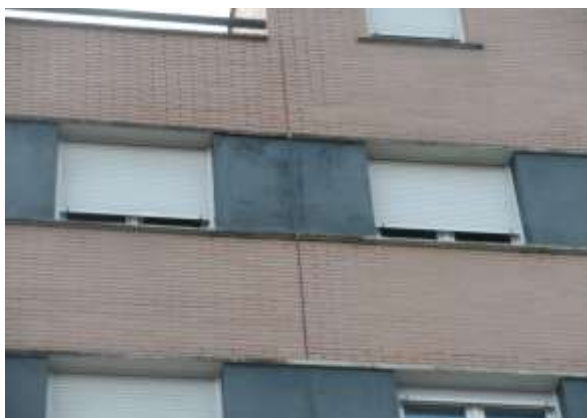
Figure 63 - Pathologies caused at the façade.
