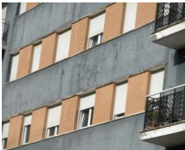
Figure 65 - Pathologies caused at the façade (3).
