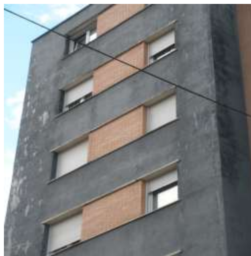
Figure 66 - Pathologies caused at the façade (4).
